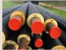
District Heat System
